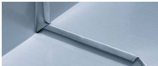
Pinched seam on roof penetration (2) Front area
