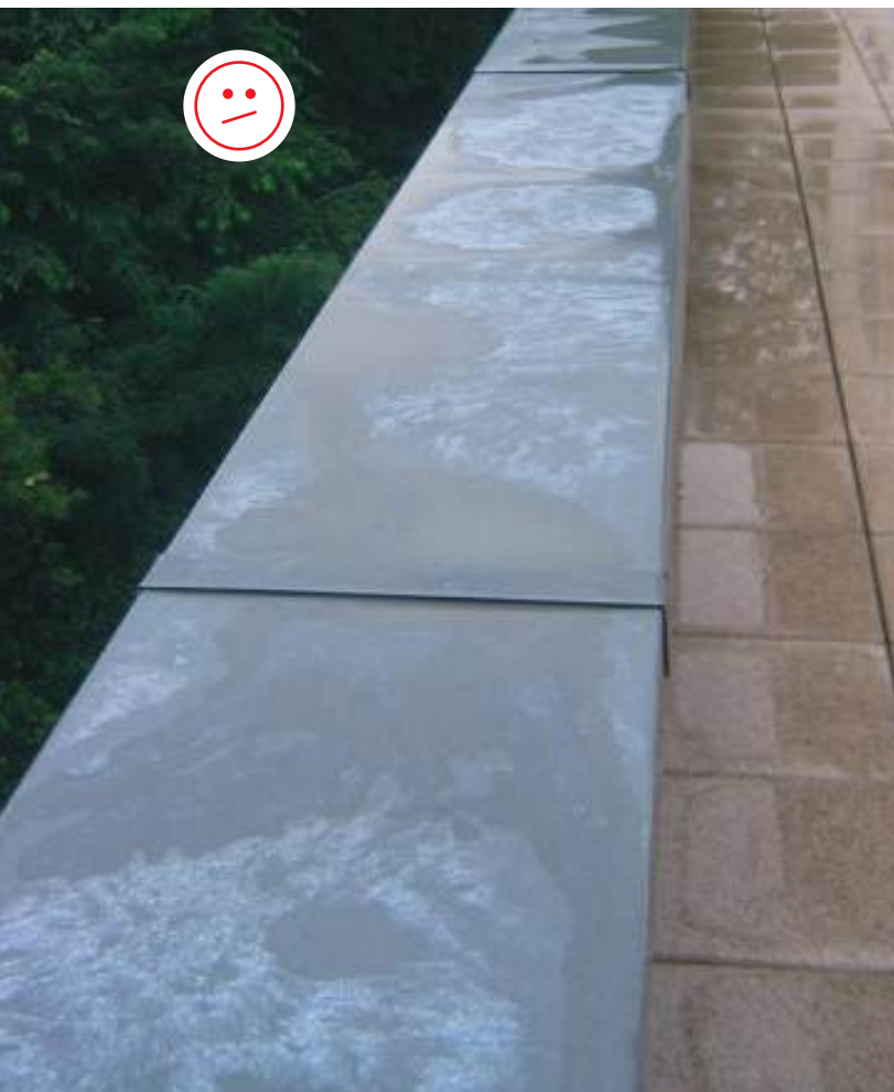
Zinc hydroxide formation due to insufficient slope
